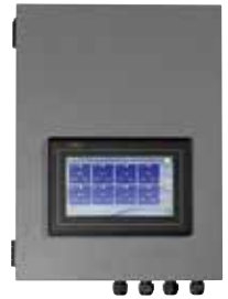
Single remote control screen in the equipment room for controlling several units (optional) Code : AO1500001
